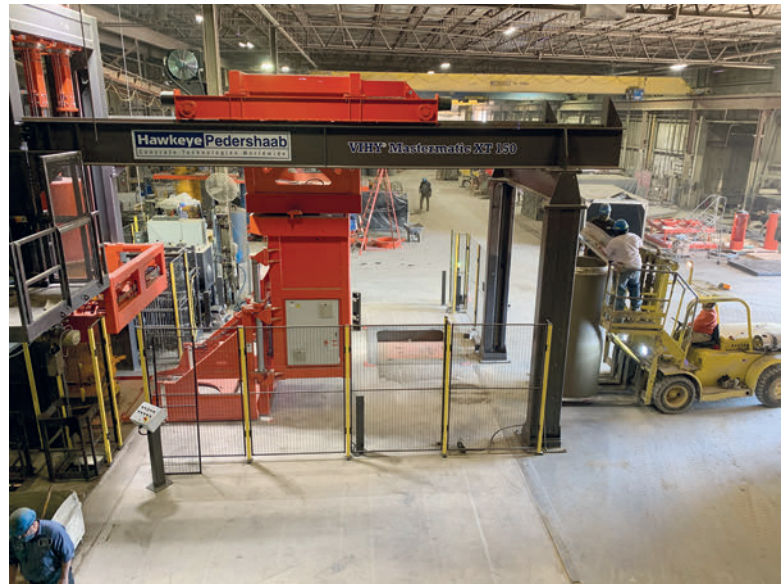
Newly installed HawkeyePedershaab Mastermatic XT150 at Northern Concrete Pipe's Grand Rapids, MI, plant.
