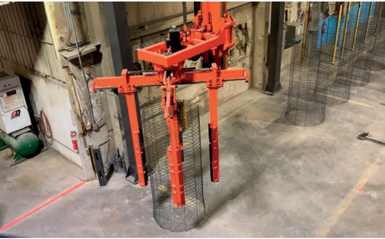
The automatic cage handling system saves labor and reduces safety risks from manually moving and lifting cages.
