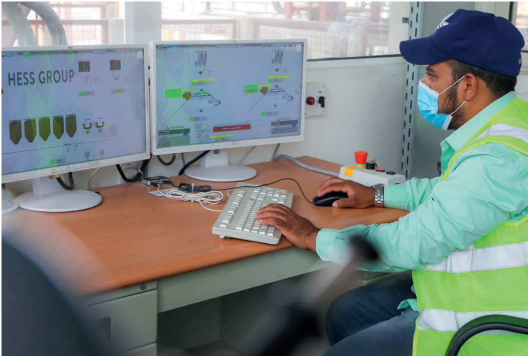
Mixing plant control
