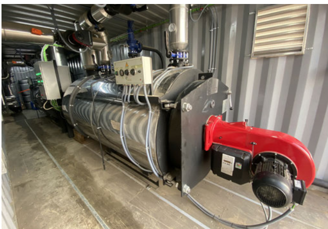
Boiler equipment with capacity of 2 x 800kW per hour in containers
