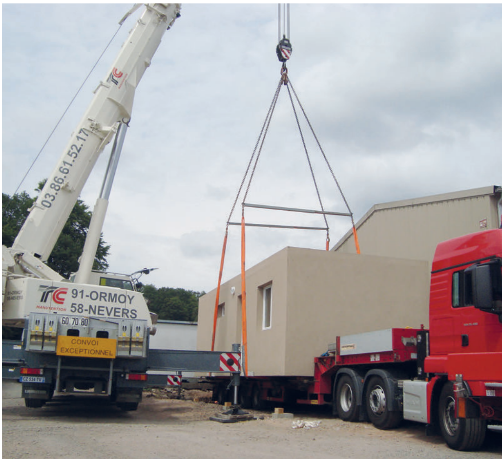
Positioning a modular Cubik Home with Dramix fibre reinforced concrete at its final location
