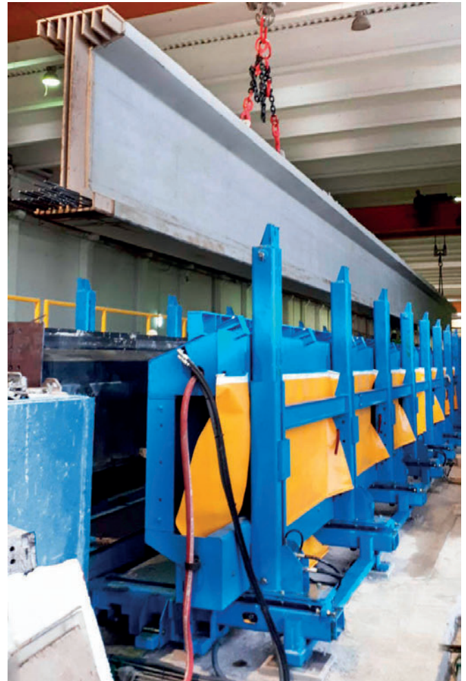
Removing a concreted beam from the variable mould with individually adjustable sections
