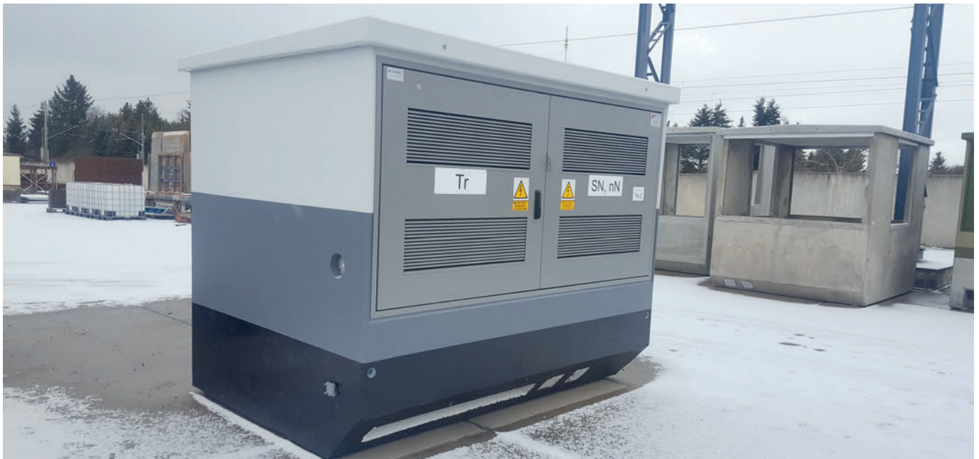
Example of a finished substation
