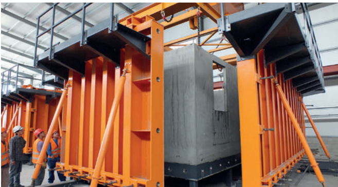
For production in installation position, the 35 t shrinking core is placed inside the mould for casting and lifted out for demoulding.
