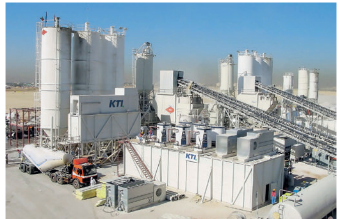
Concrete cooling systems made by KTI-Plersch Kältetechnik GmbH for generating a total of 2.6 million m 3 of cooled concrete. These were employed in the construction of Dubai International Airport
