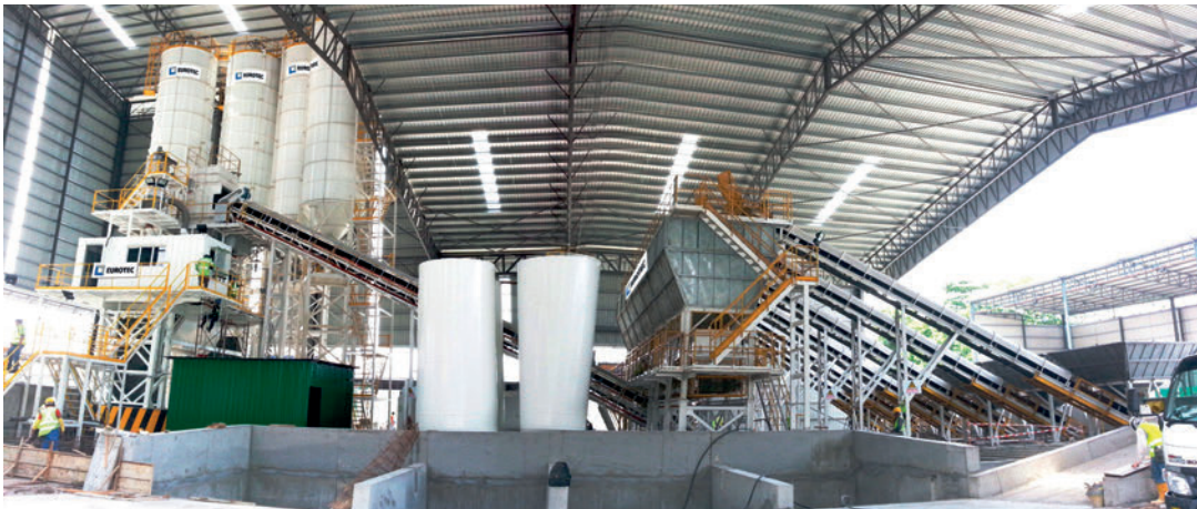
Eurotec MZP200 ready mix concrete batching plant installed within an enclosed warehouse
