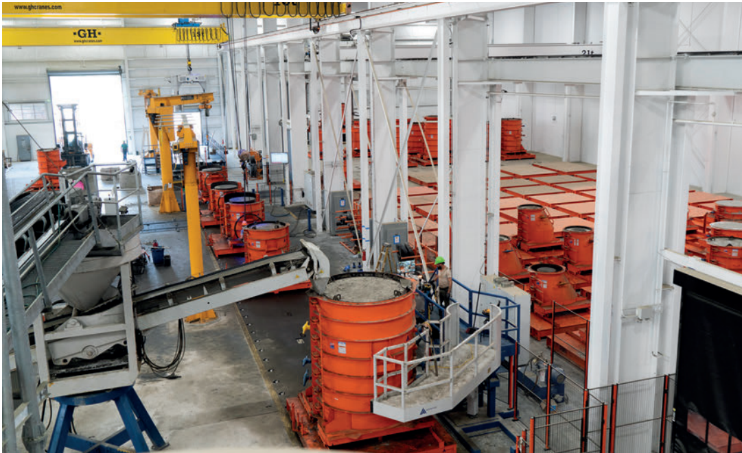
The Prima process line at the new Tindall plant in Spartanburg, SC.
