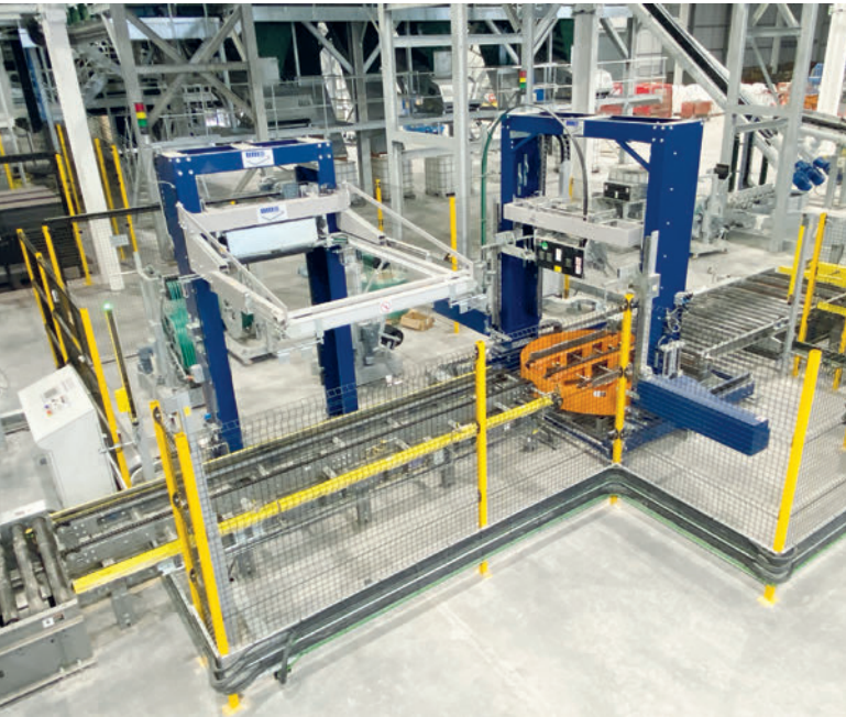
The first of two sets of horizontal and vertical OMS strapping machines.
