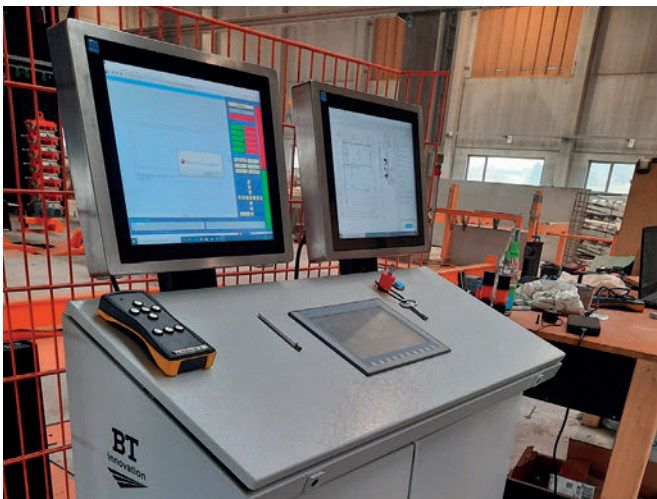
Control point for unfolding and folding station and laser projectors
