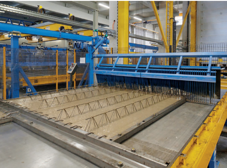
Pallet transport to the storage and retrieval machine
