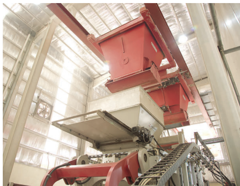
The double bucket conveyor transfers the core and facing concrete into the concrete block machine's corresponding storage silos.
