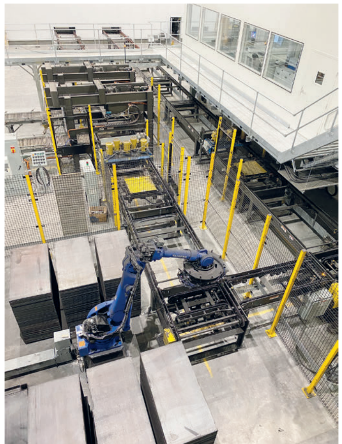
Twin dry side pallet return, lift blade push-offs, brush, grinding and pallet turn-over to robotic buffer accumulation of 510 pallets.
