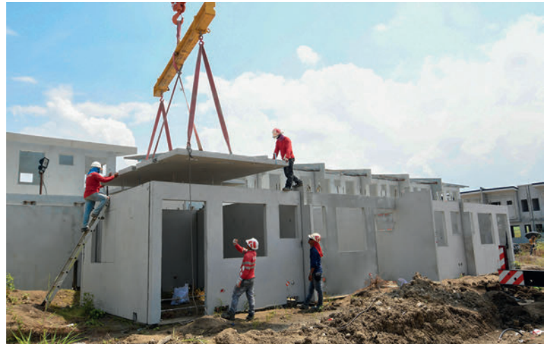
The precast elements used are 100 mm wide solid walls all around both floors as per minimum code requirement. The 120 mm solid slabs are provided as one piece.
