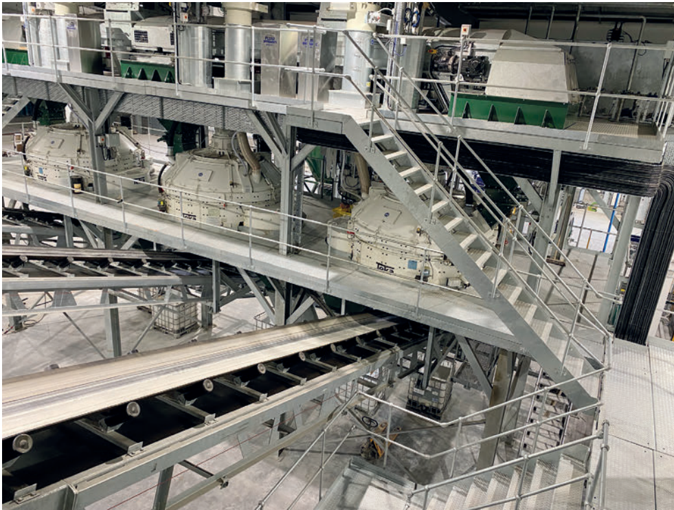
Plant mixer station by Concrete Batching Systems, Ireland.
