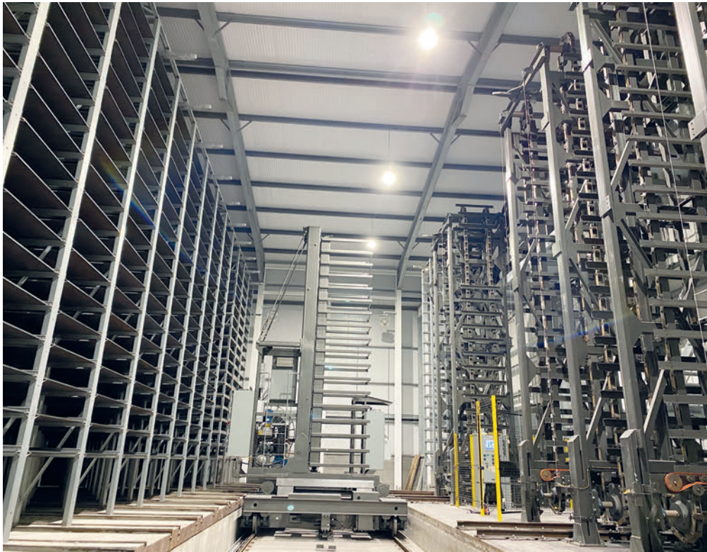
Columbia 18 tonne PTS with turntable, green side stacker, 2 x buffers, 2 x dry side unstackers + CDS chamber racking system for 7,000 pallet capacity.
