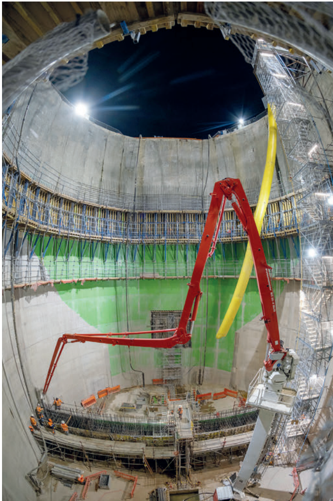
Agru supplies Ultra Grip concrete protective liners for the largest wastewater project in New Zealand's history.
