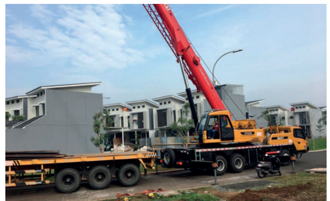
The building time is enormously reduced by building with prefabricated elements that are installed on site with cranes and qualified staff.
