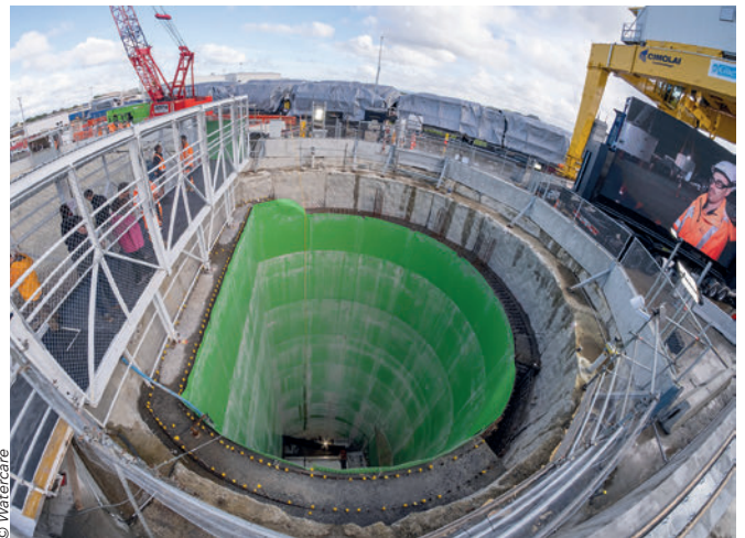
The access shaft is protected from concrete corrosion with green Ultra Grip concrete protective liners.
