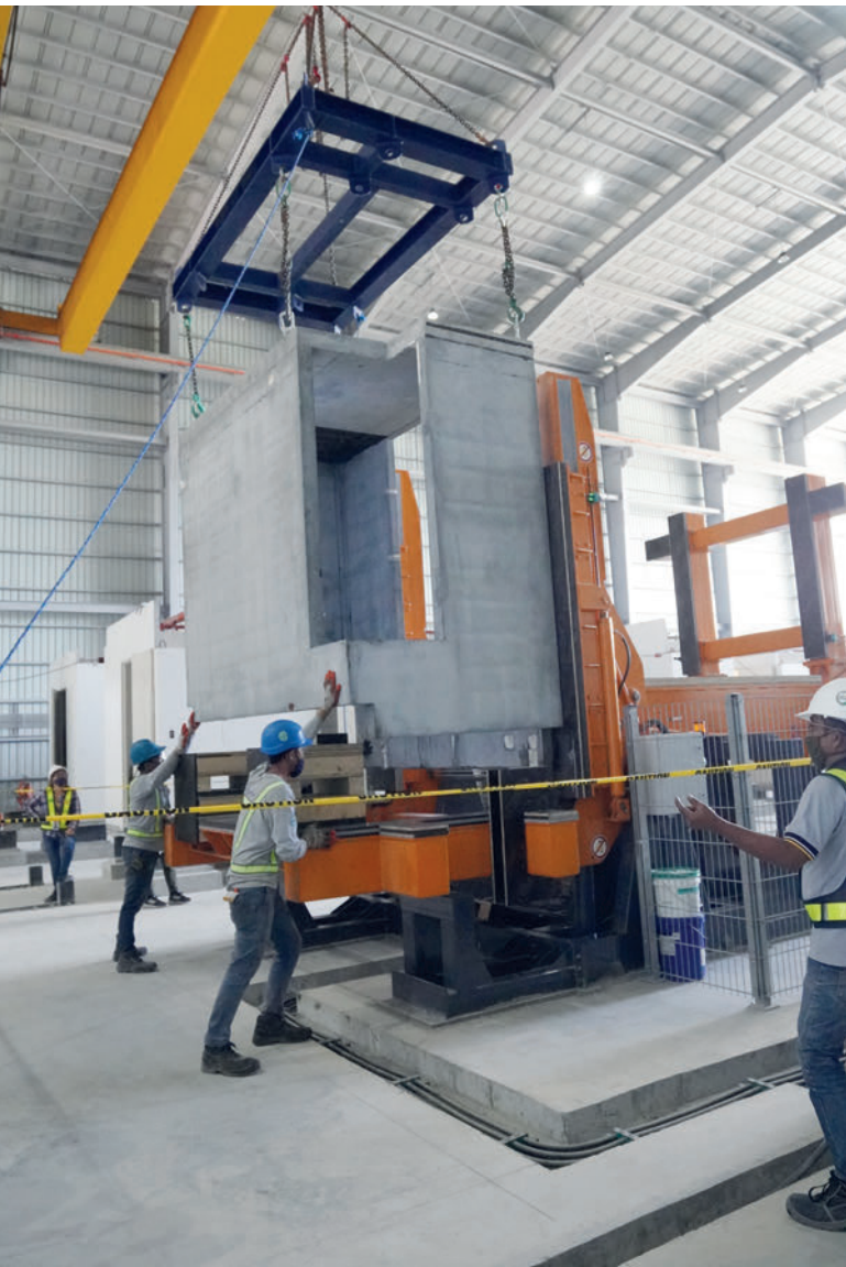
A turning unit was part of the scope of supply.
