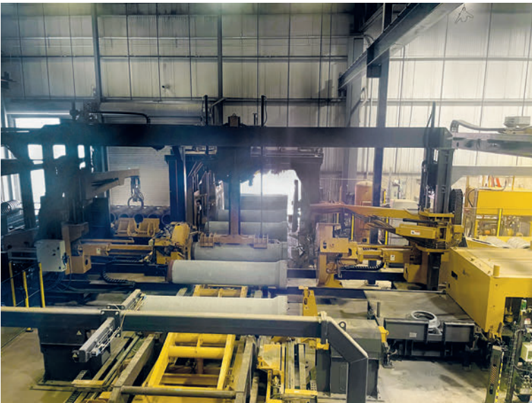
Afinitas Roco system layout at the Oldcastle Infrastructure pipe plant in Ogden, UT.
