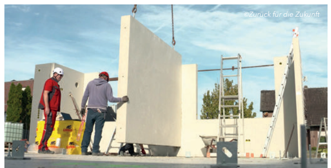
Assembly of the environmentally friendly concrete components from the Büscher concrete plant.
