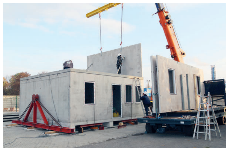
Processing of elements smooth on all sides as room module components on the construction site.
