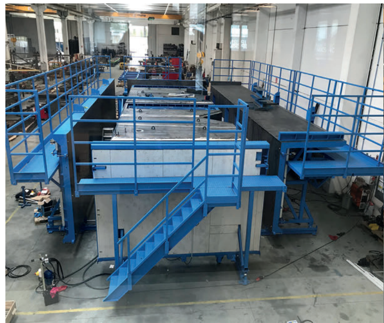
Commissioning at Construx of a quadruple cell mould before going to Melbourne, Australia
