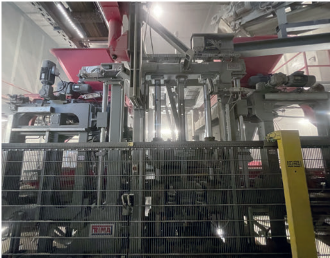
Frima HP1000 in use at Egner's Erasbach plant in Germany.
