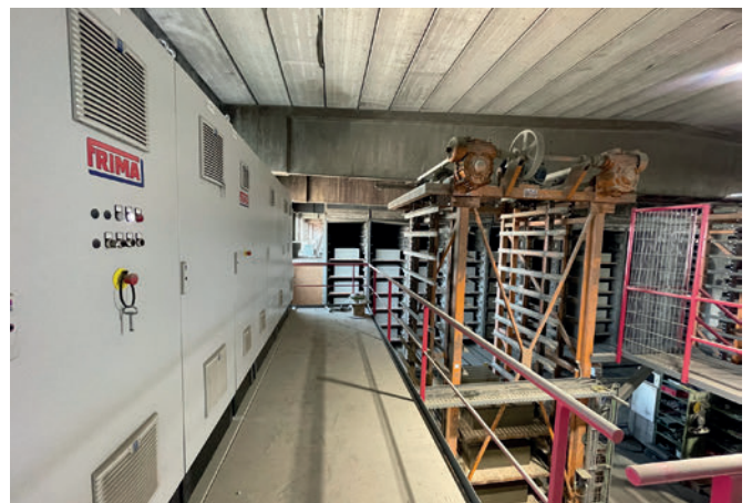
The control cabinets are located on the upper level.
