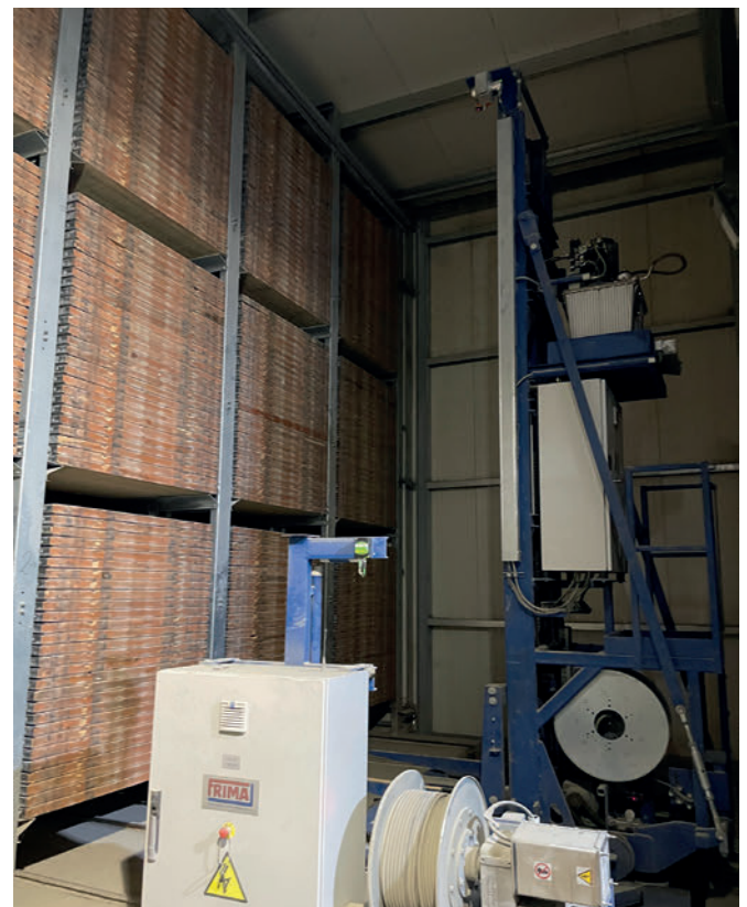
Board packaging vehicle assembly with turntable for buffering board packages over three floors.
