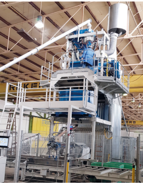
Fully automatic industrial Sandosit production plant
