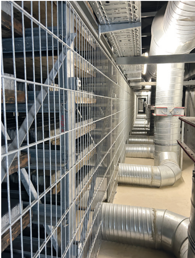
The air is distributed evenly and precisely in the chamber through a technical duct system.
