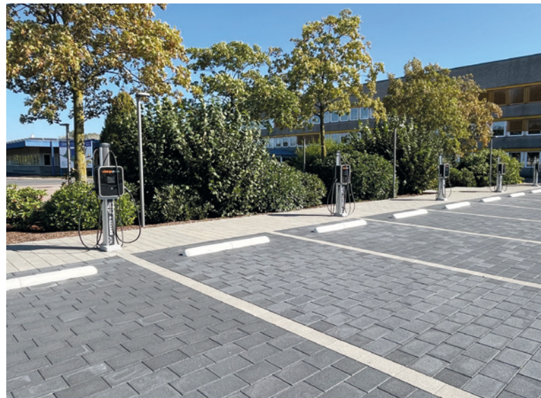
Rekers e-parking for employees and customers
