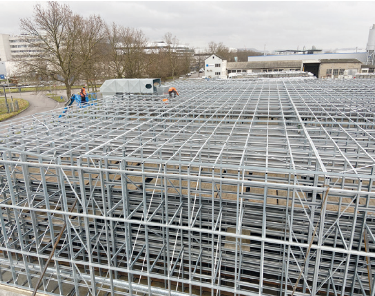
HS Anlagentechnik has installed an outdoor version of a large chamber system with 21 aisles and 16 shelves.
