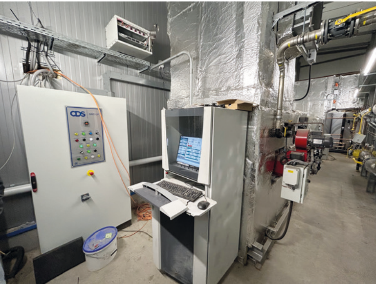
The Envirocure system works with a highly efficient 450 kW gas burner.
