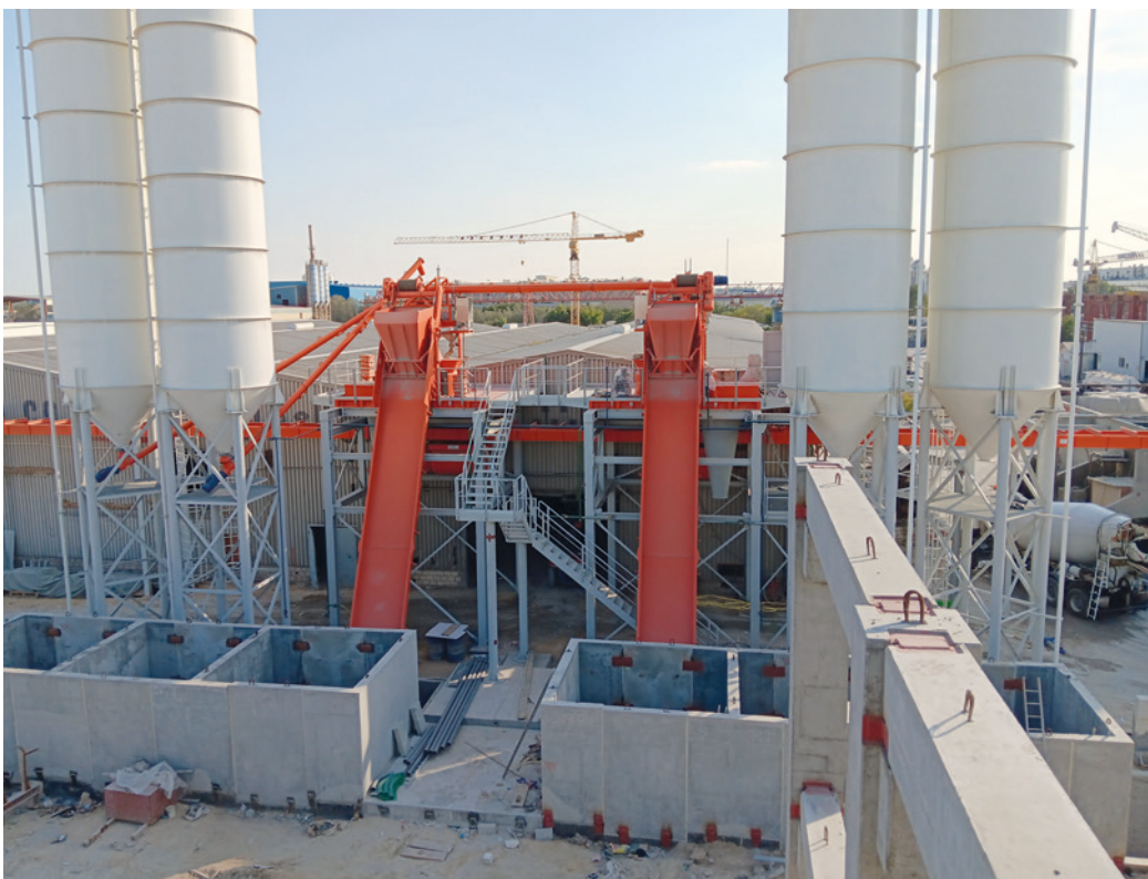
Two HPGM with skiphoists and six aggregate bins
