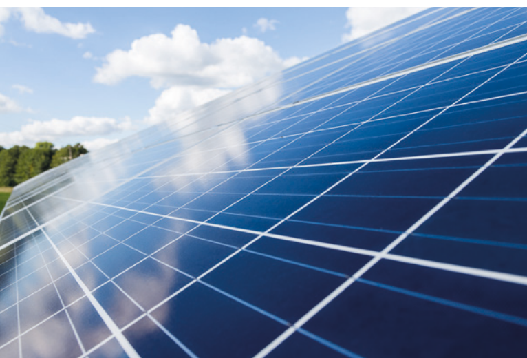
With the current expansion of the photovoltaic system, approx. 2.3 MWh of solar power is already available
