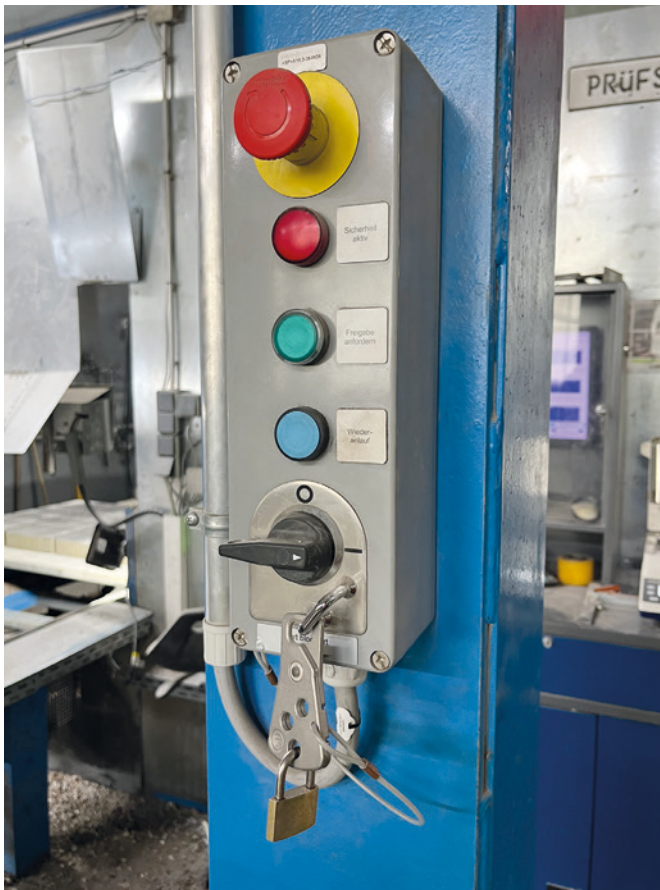
Safe and practical: Lockout-Tagout maintenance protection
