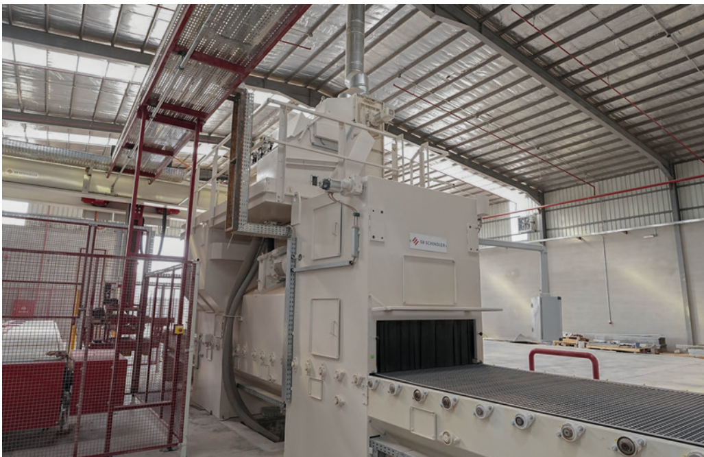
Shotblasting unit (in commissioning)
