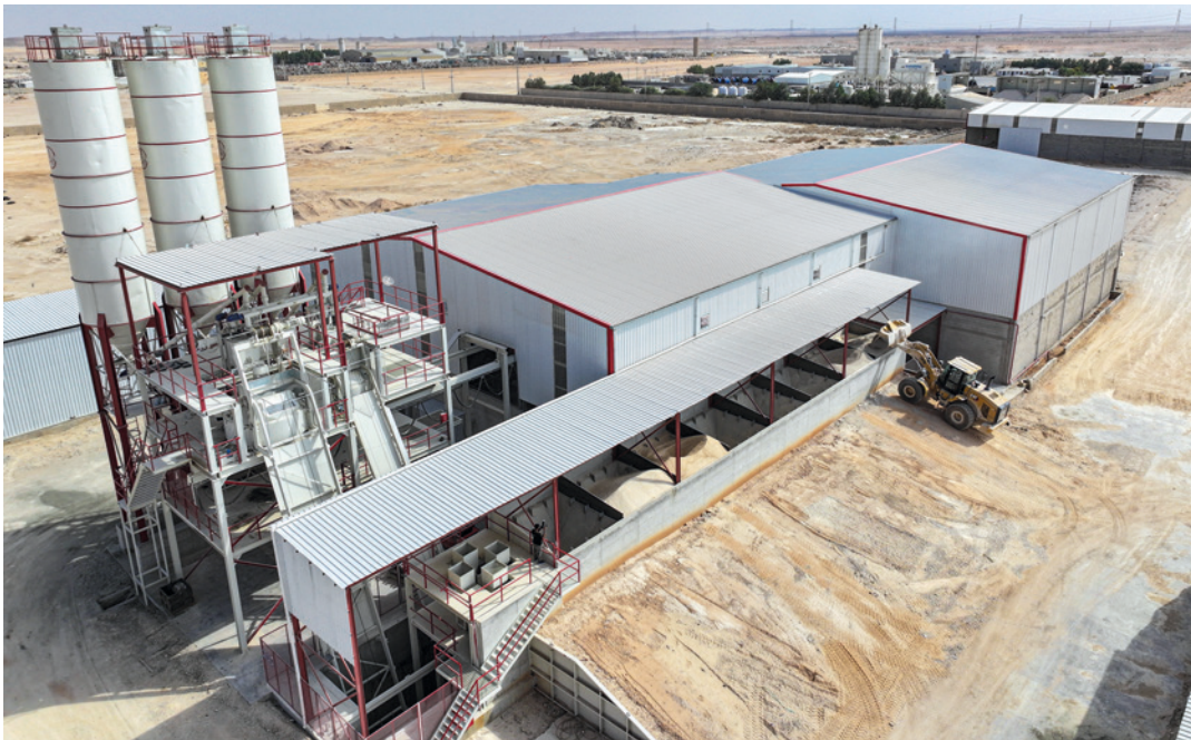
Outside view of the OTC plant
