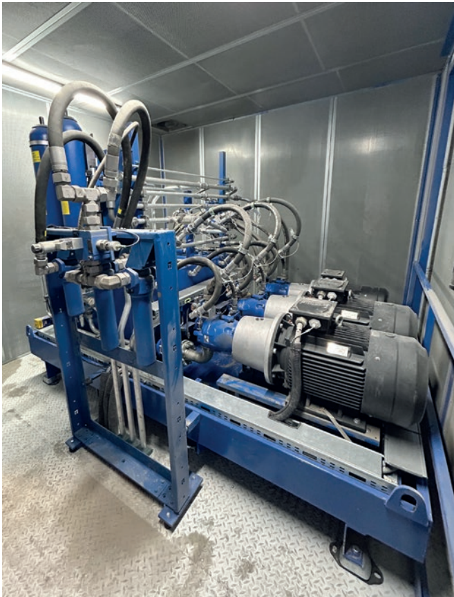
High-performance hydraulics in a separate hydraulic room.
