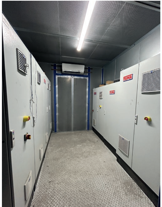
Air-conditioned control cabinet room.
