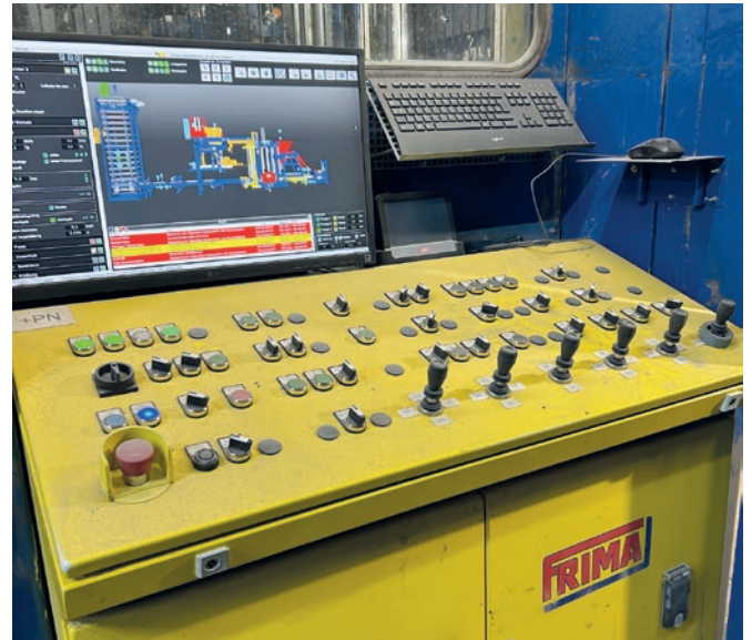
Control panel and visualization of the system.
